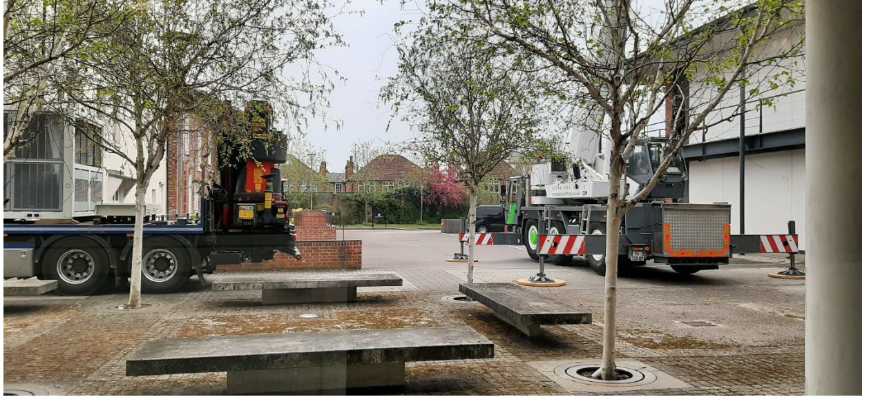
A significant investment: after 21 years of service by our old air-conditioning chiller, a new one (left) arrives to replace it (see page 20)
